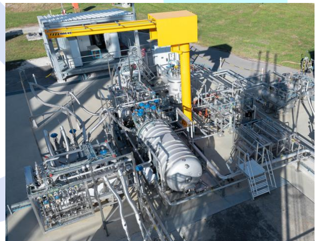
Fig. 2: Similar LH2 tank test installation (Credit: Airbus - for illustration only)
